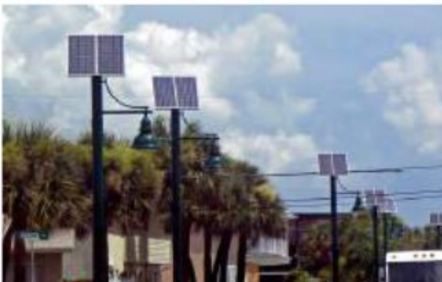
Solar Powered Lighting | Cape Canaveral, FL
